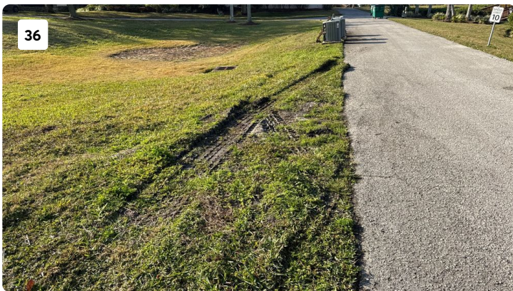
Vehicle traffic should be kept on the roadway, this was discussed with SWR
