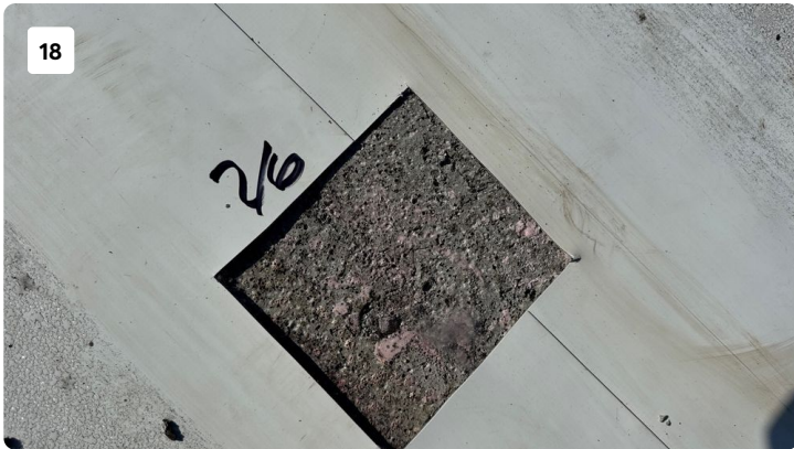
adhesive is light at the seams. contractor to let foam rise and set up more prior to rolling in the sheet at the seams.
