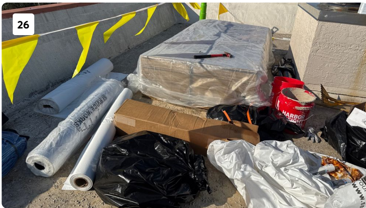
Plywood is on site and properly stored in case replacement of the walls are needed
