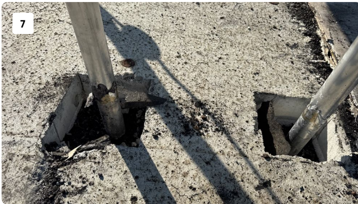
showing stands are cut into the LWC and are mounted to the structural concrete.
