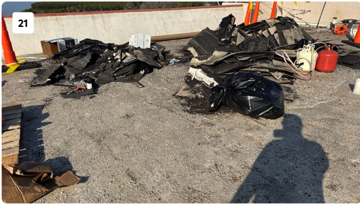
21 Trash is being stockpiled until it can be downloaded into the dumpster shoot.
