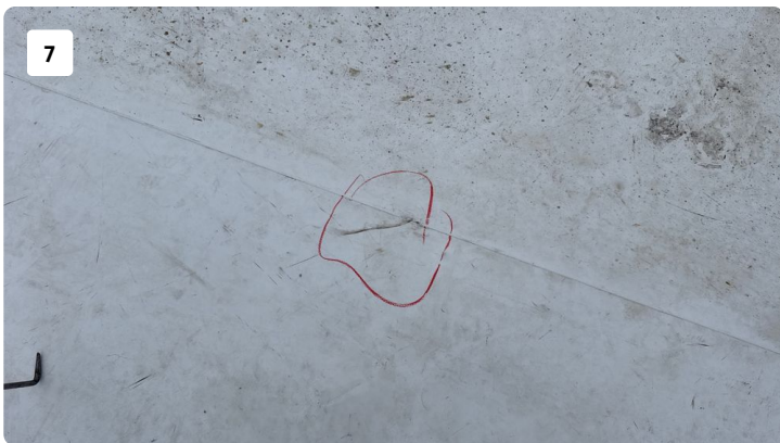
Cut in the laps seam to be properly patched.
