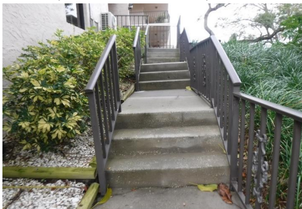
7 Uneven Stairs due to settlement
