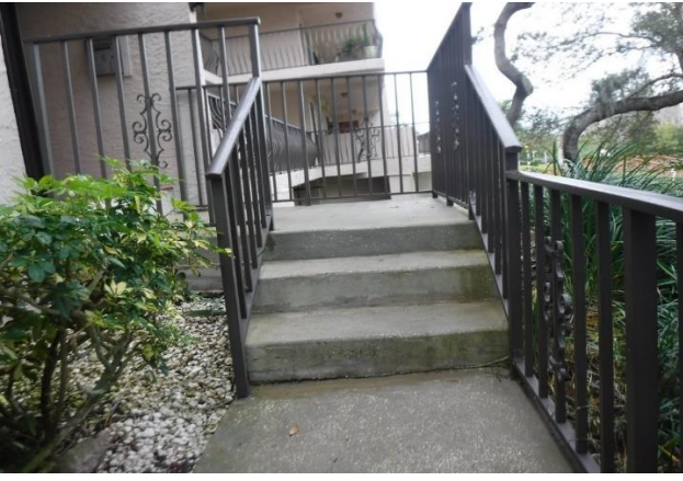
9 Uneven Stairs due to settlement
