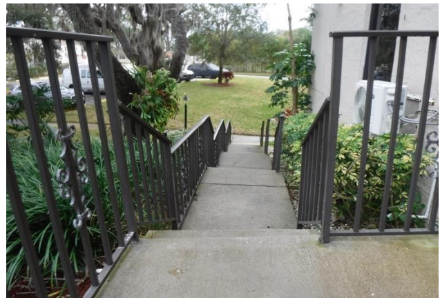
6 Uneven Stairs due to settlement
