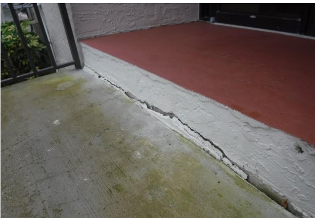
5 Separation at the front Stoop
