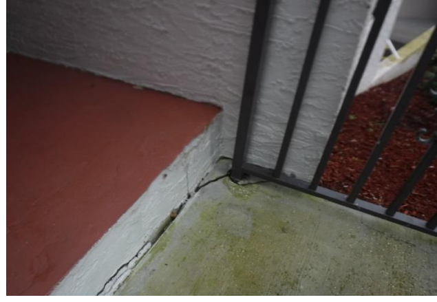
10 Separation at the front Stoop
