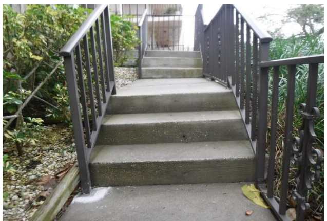
8 Uneven Stairs due to settlement
