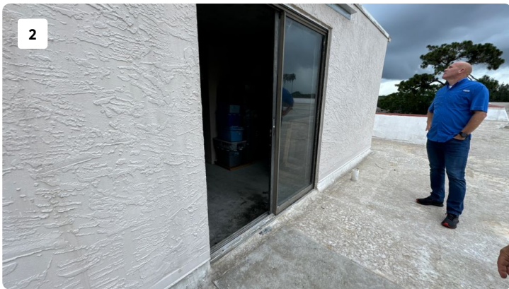
door to be replaced.
