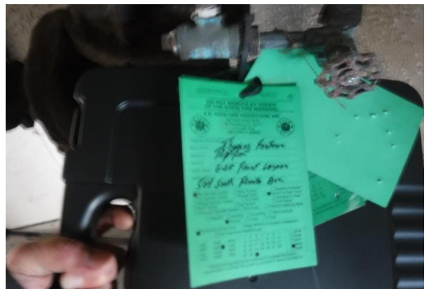
36 Bldg. #502 Backflow Preventer Overview
