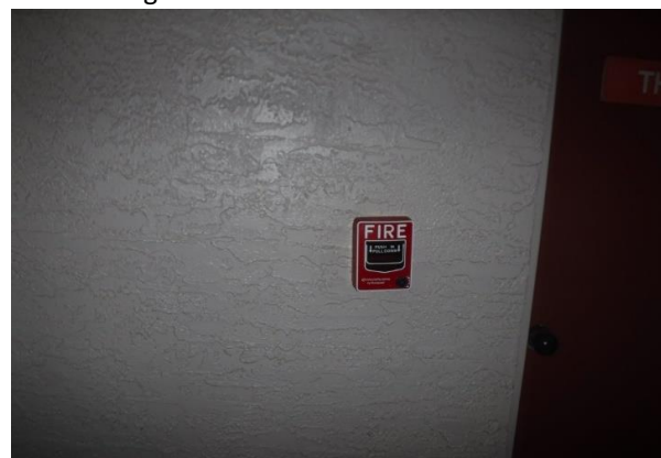
30 Bldg. #502 Fire Alarm Overview
