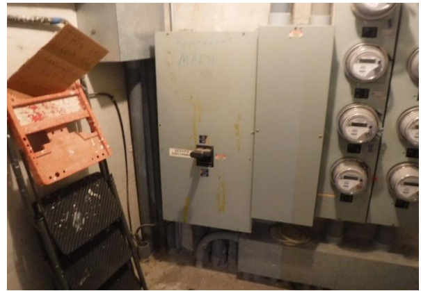
92 Building #504 Electrical Main Overview
