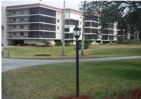
113 Building #504 Lighting Overview
