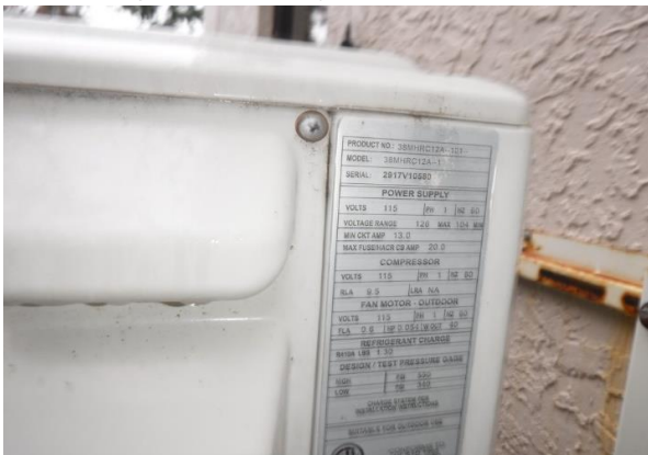
55 Bldg. #502 HVAC Split Data Plate
