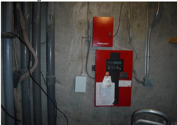
29 Bldg. #502 Fire Alarm Overview
