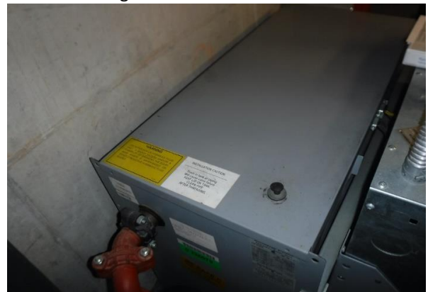
90 Building #504 Elevator Motor Overview
