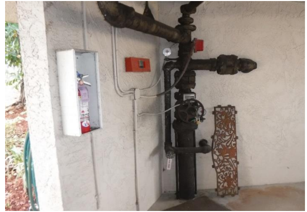
96 Building #504 Main Water Valve Overview
