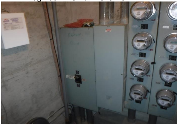
31 Bldg. #502 Electrical Main Overview
