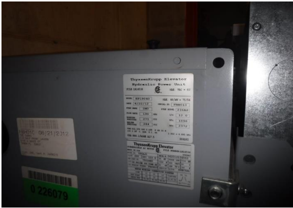
91 Building #504 Elevator Motor Data Plate
