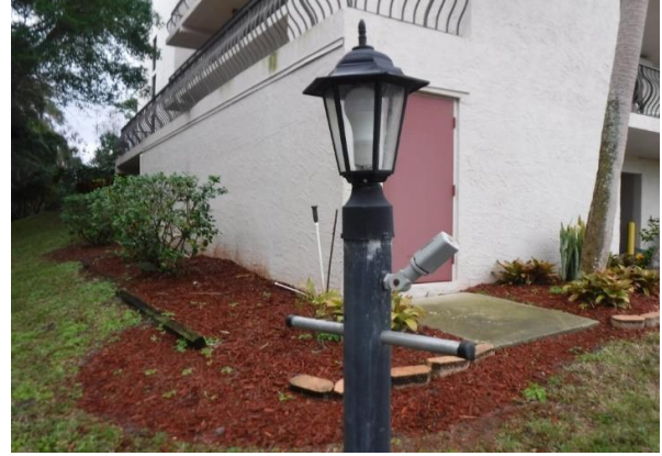
52 Bldg. #502 Lighting Overview
