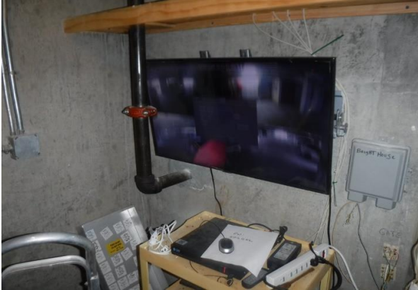
59 Bldg. #502 Security System Overview
