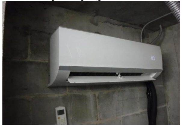
114 Building #504 HVAC Split Overview
