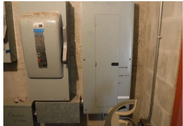
94 Building #504 Electrical Subs Overview
