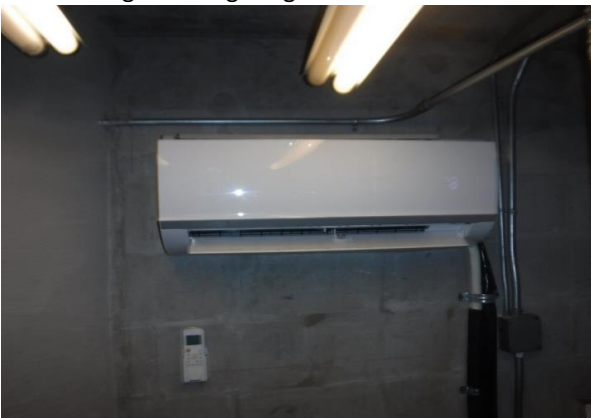
53 Bldg. #502 HVAC Split Overview
