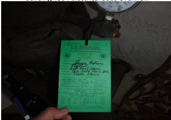
97 Building #504 Backflow Preventer Overview
