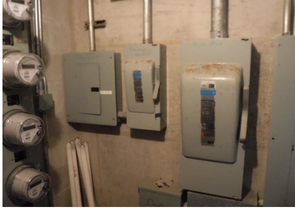
93 Building #504 Electrical Subs Overview
