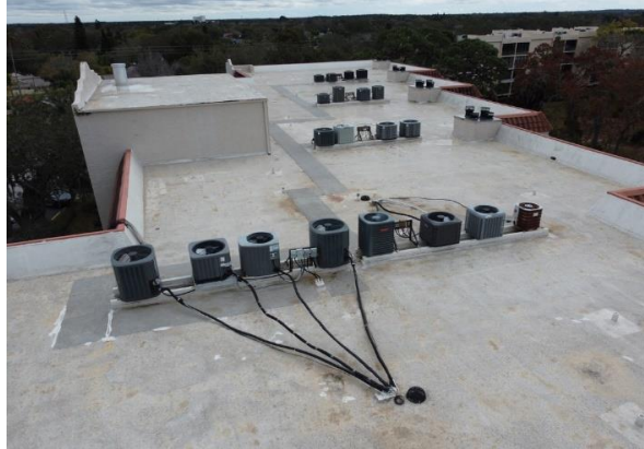
77 Building #504 HVAC Stands Overview
