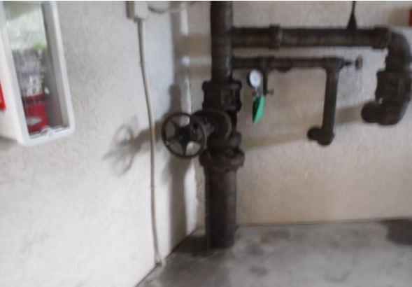
35 Bldg. #502 Main Water Valve Overview
