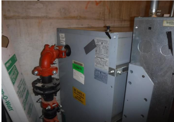
27 Bldg. #502 Elevator Motor Overview
