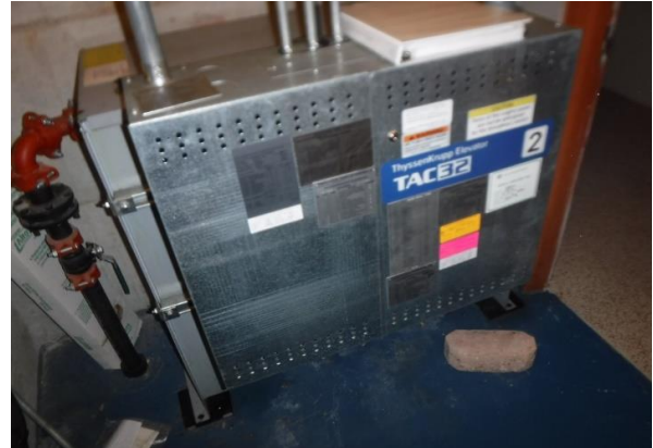
26 Bldg. #502 Elevator Control Panel Overview
