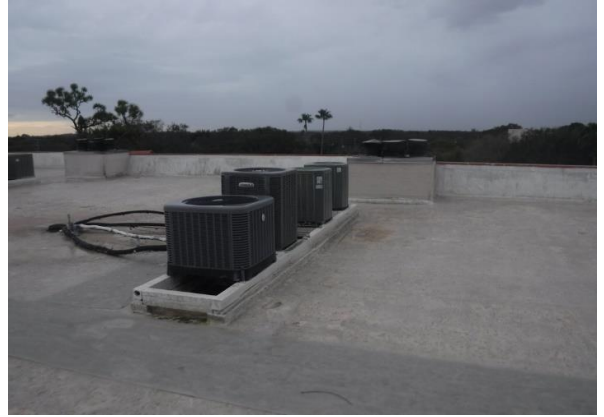
12 Bldg. #502 HVAC Stands Overview
