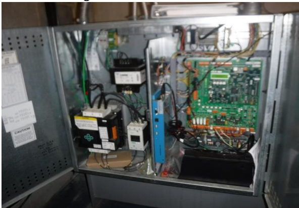
89 Building #504 Elevator Control Board Overview
