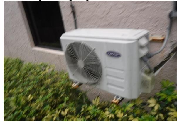
54 Bldg. #502 HVAC Split Overview
