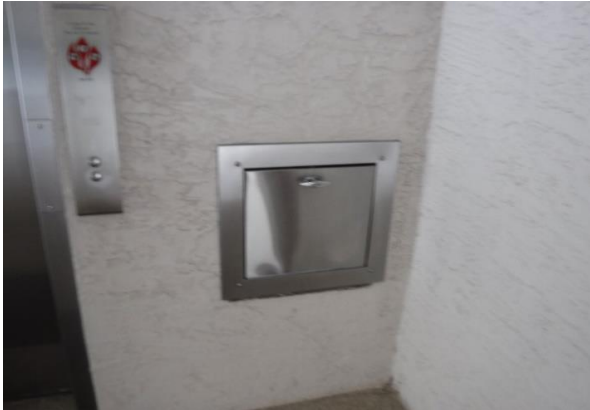
117 Building #504 Trash Chute
