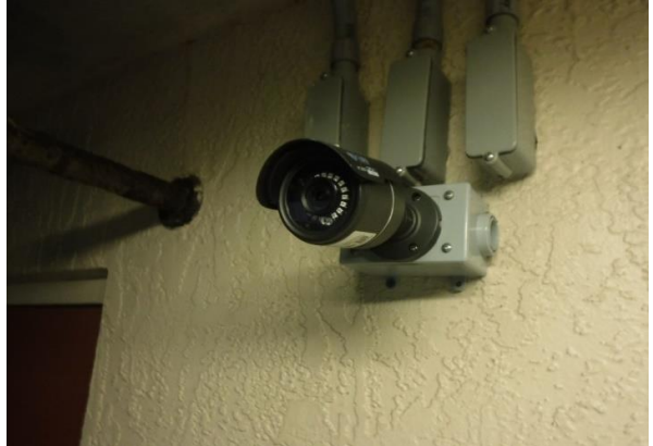
60 Bldg. #502 Security System Overview
