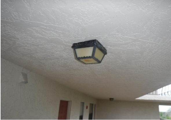
51 Bldg. #502 Lighting Overview
