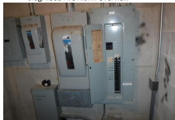
32 Bldg. #502 Electrical Sub Overview
