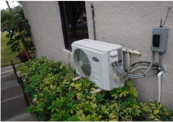
115 Building #504 HVAC Split Overview
