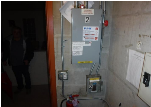
33 Bldg. #502 Electrical Sub Overview
