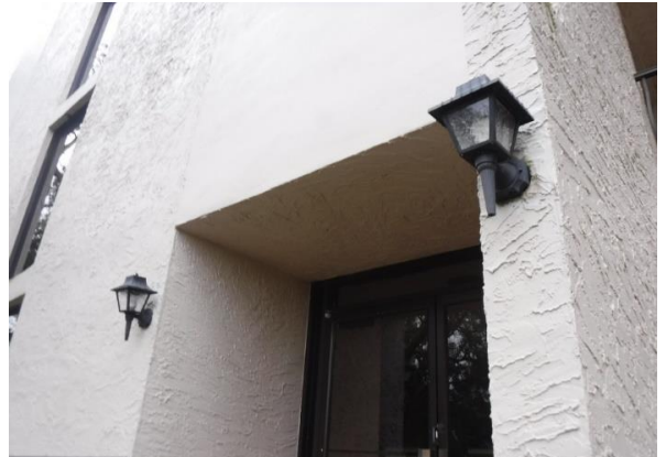
112 Building #504 Lighting Overview
