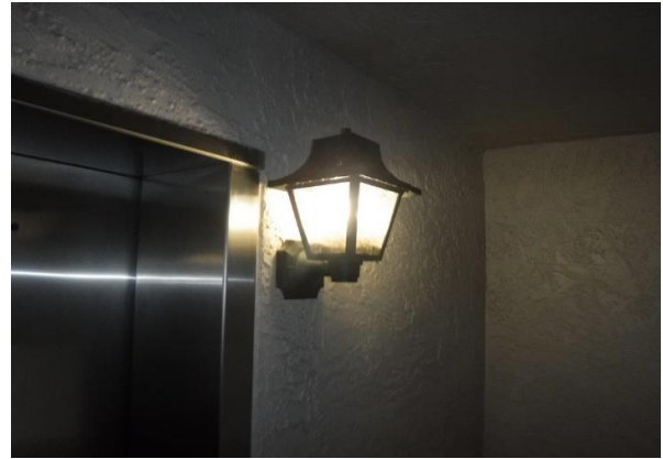
50 Bldg. #502 Lighting Overview
