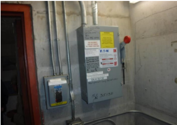
95 Building #504 Electrical Subs Overview
